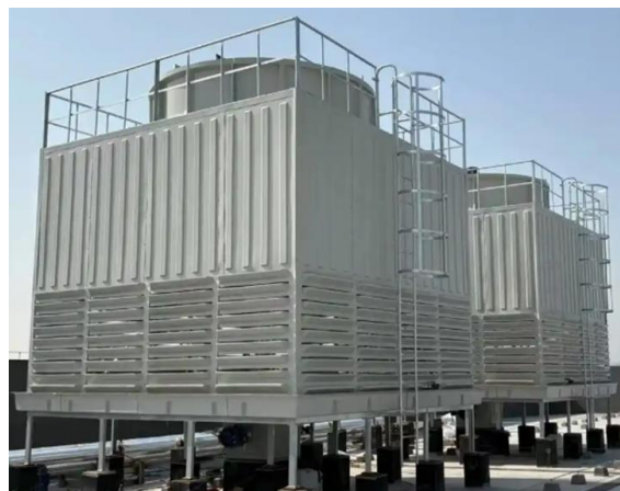
냉각탑 cooling tower
